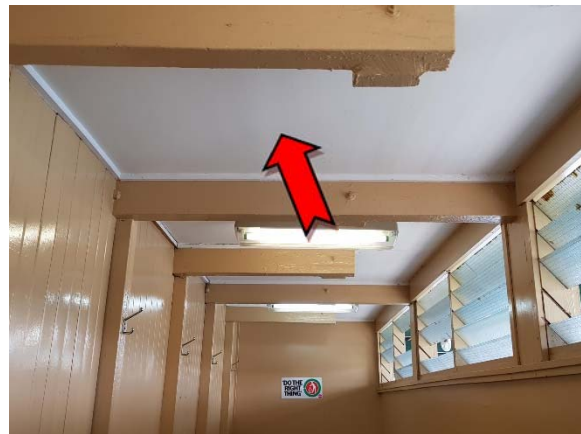
Photo 4. Interior, female change rooms, ceiling – asbestos-containing fibre cement sheeting.
