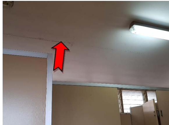
Photo 10. Interior, men's change room, ceiling – asbestos-containing fibre cement sheeting.
