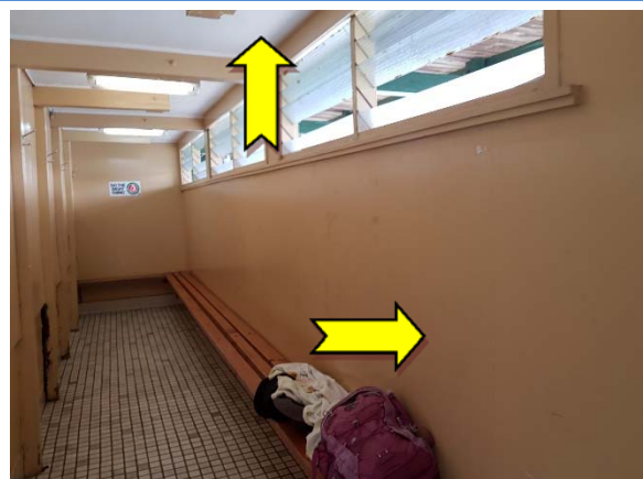
Photo 18. Interior, throughout, walls and ceilings – suspected lead-containing yellow and white upper coloured paint systems.
