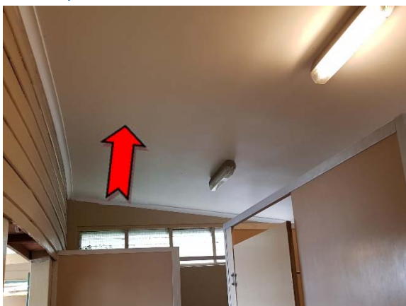
Photo 11. Interior, men's toilets/showers, ceiling – asbestos-containing fibre cement sheeting.
