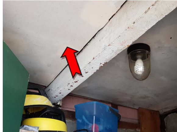
Photo 8. Interior, store room, ceiling – asbestos-containing fibre cement sheeting.
