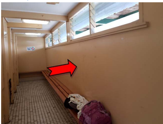
Photo 5. Interior, female change rooms, wall – asbestos-containing fibre cement sheeting.
