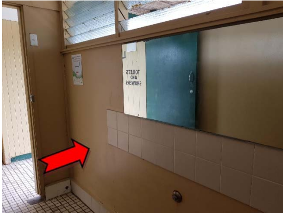
Photo 7. Interior, ladies toilets/showers, wall – asbestos-containing fibre cement sheeting.
