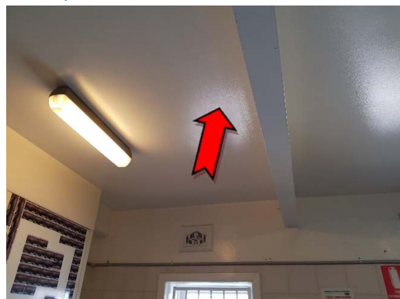
Photo 6. Interior, ladies toilets/showers, ceiling – asbestos-containing fibre cement sheeting.
