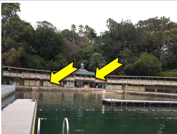
Photo 17. Exterior, throughout, walls and beams – suspected lead-containing yellow and green upper coloured paint systems.
