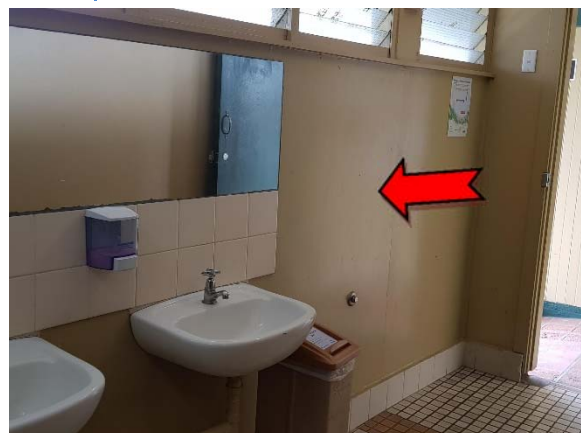
Photo 12. Interior, men's toilets/showers, wall – asbestos-containing fibre cement sheeting.
