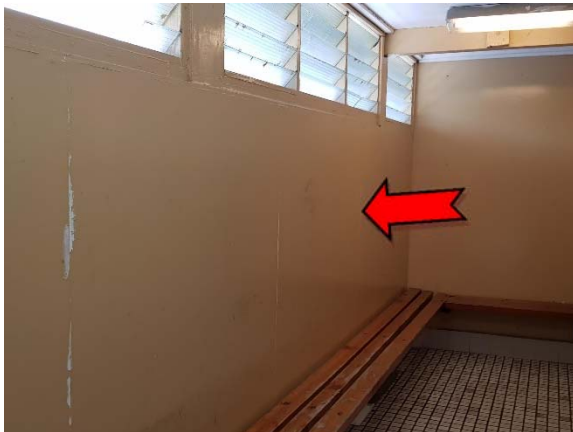
Photo 9. Interior, men's change room, wall – asbestos-containing fibre cement sheeting.
